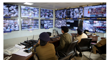
Centralized Control Room
